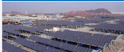
Seonam Municipal Wastewater Treatment Plant, (2,995 kW) Completed in Feb. 2014
