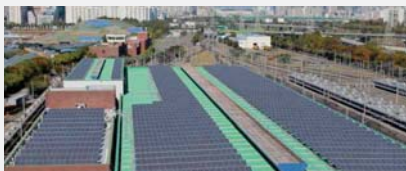
Suseo Train Depot (700 kW) Completed in Nov. 2013
