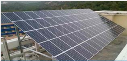
Bukhansan Hillstate Apt III, PV 20kW
